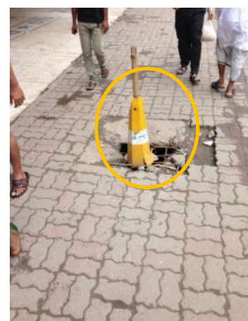
Broken drainage cover
