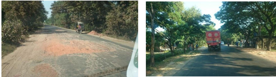
Figure 4.47 Existing Condition of Highways (Dhaka Bypass)
