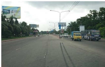
Worn-out lane marks
